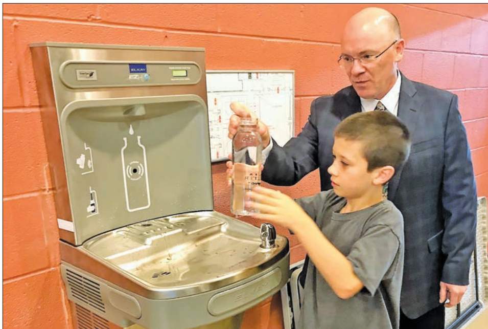
Derry Township-based Pennsylvania American Water donated a water bottle filling station to The Vista School in Derry Township to decrease environmental waste and improve health and wellness for students and staff. The Vista School serves more than 100 children with autism from eight counties, from pre-kindergarten to secondary school age. Shown above, Pennsylvania American Water Vice President of Operations Jimmy Sheridan and a student use the new water station in the school's gym.
