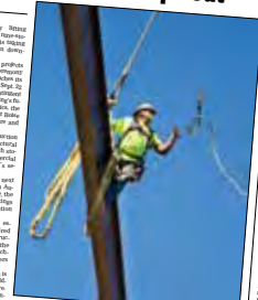
Retief says a rafter is raising the final steel beam at the City Center Plaza building in downtown Boise.
