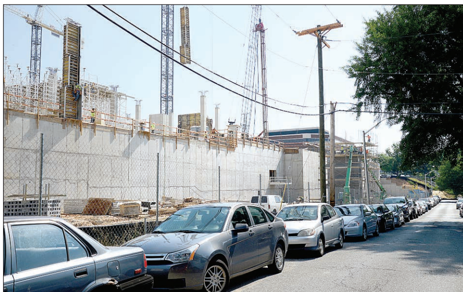
The construction at the Rotunda on 40th Street has led to a proposal to restrict parking. A sign points to where customers should park while they patronize businesses in Hampden Village. Cars line 38th Street behind the construction site.
