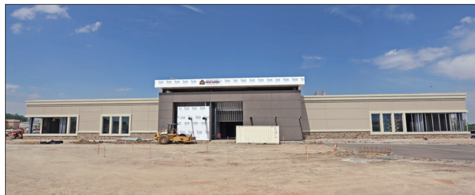
Construction continues on the Ashley Furniture showroom at the Tulsa Hills Shopping Center in west Tulsa. PHOTO BY RIP STELL
