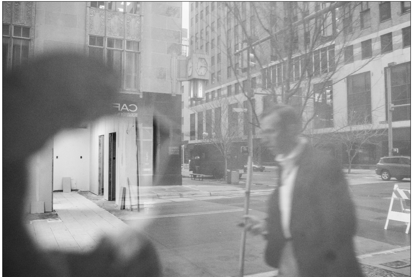
The retail space in the northwest corner of the Robinson Renaissance is under renovation. Paper covering the windows hides ongoing work, but a small tear reveals a glimpse inside. PHOTO BY BRENT FUCHS
