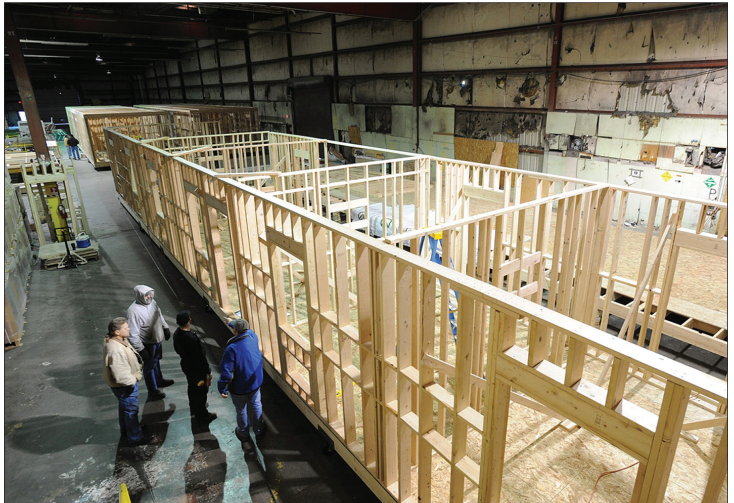
System Building Solutions workers work on a 20-room modular building in the former Boise Cascade factory in Laurel, Mont. AP PHOTO
